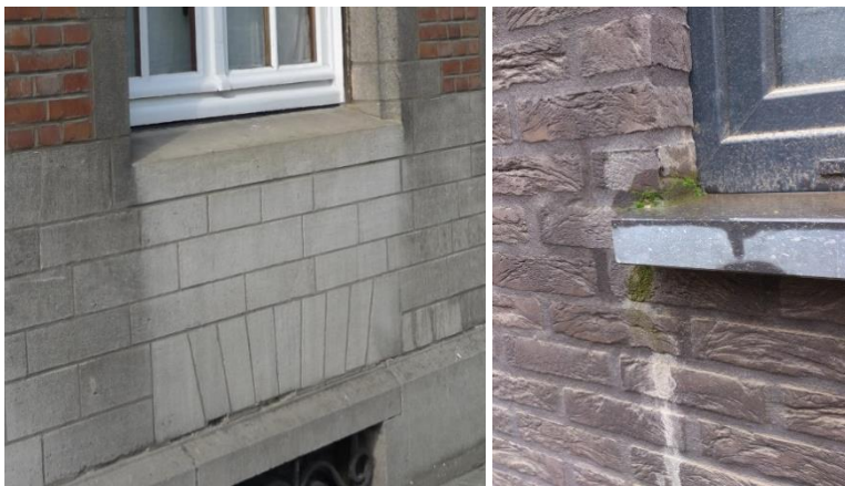
Fig. 7 Unfavourable design: window sill does not protrude from the façade (left) or no edging of the window sill (right), so that rain can penetrate directly into the façade and cause damage.
