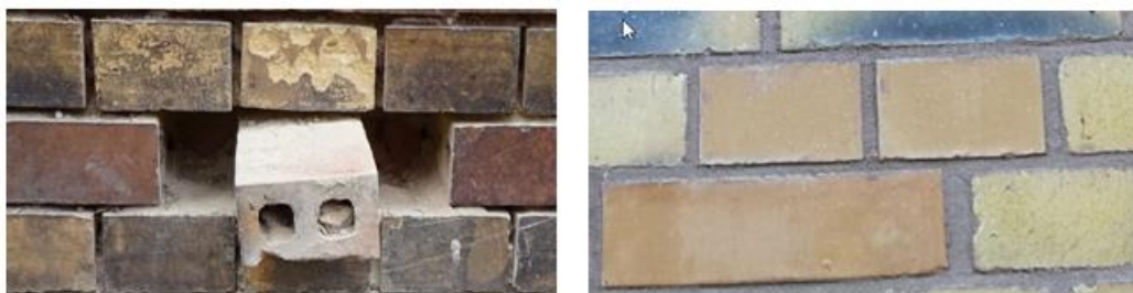
Fig. 8 Existing horizontally perforated brick in the façade: left photo during the as-built analysis, right photo after renovation
