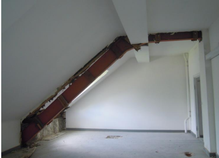
Fig. 21 Steel frame construction in the thermal plane with integration into the reinforced concrete jamb
