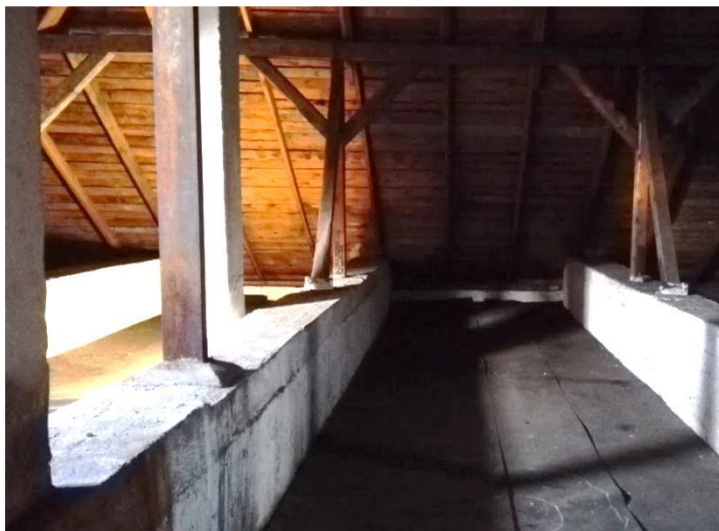
Fig. 20 Example of a reinforced concrete overlay in the ceiling to the unheated loft
