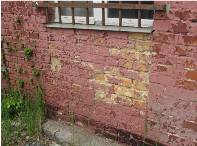
Fig. 3 Example of dense coatings to be removed
