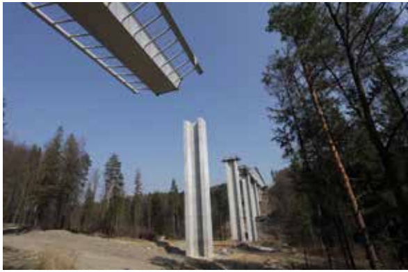
Fig. 15: Launching of the Bridge across the Kremlice Creek Valley (Photo: Jiri Dvorak)
