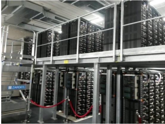
WEMAG 5MWh PCR battery storage
