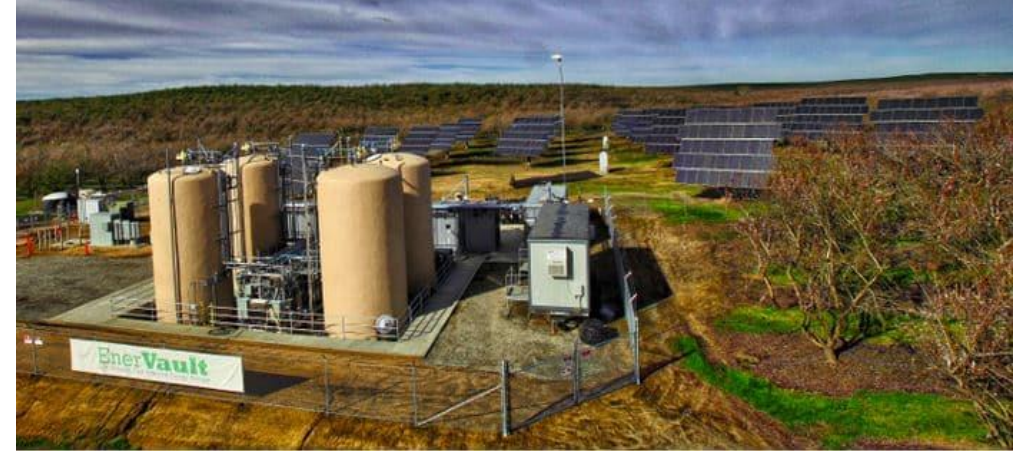
Turlock 250 kW / 1 MWh Fe/Cr RFB © EnerVault
