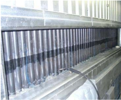
Fig. 12a. Cut-out in the insulation of a boiler for installing the constantan wires.
