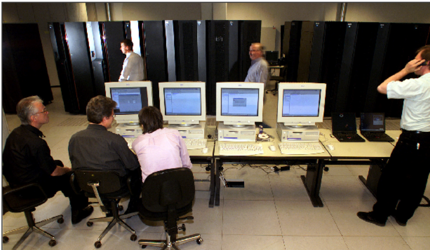
12 IBM p690 cabinets, each 4 x 8 = 32 Power4 cores, 384 cores per site
